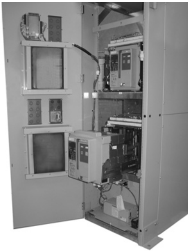
2000 Amperes, 3-Pole NEMA 1 Enclosed Drawout
