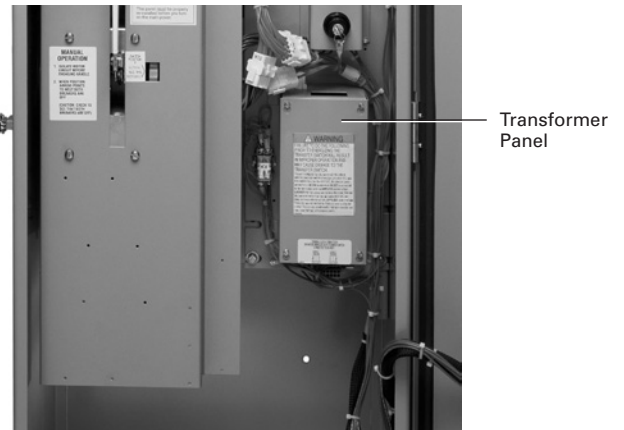
Transformer Panel Location
